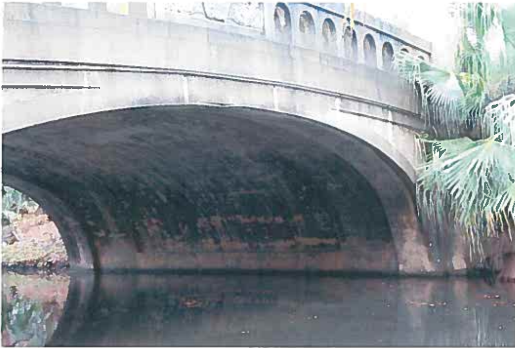
Condition Photo 12: Spalled and delaminated concrete on underside of arch of Recall No. 102227.
