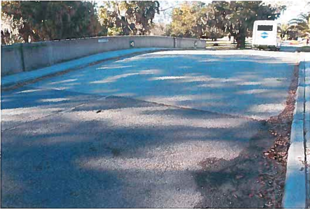
Condition Photo 10: Unsealed joints and cracks in concrete pavement over Recall No. 102226; deteriorated asphalt pavement on easterly approach roadway.
