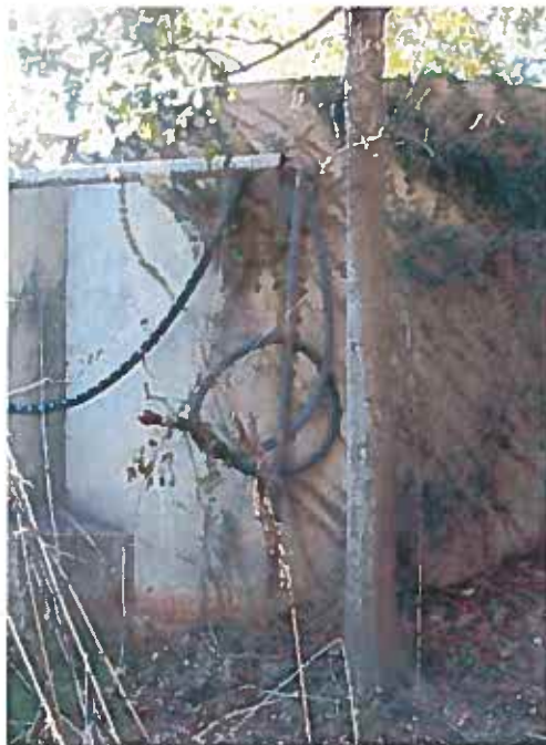
Condition Photo 7: Abandoned steel conduit and wiring on north side of Recall No. 102113.
