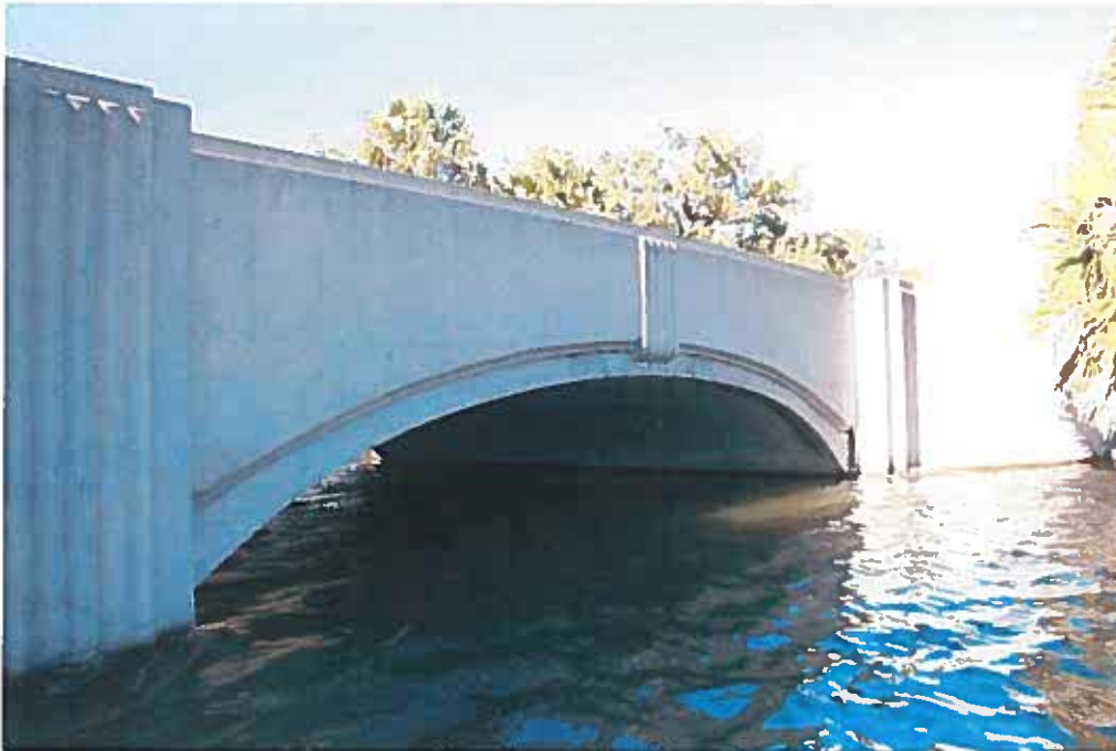
Condition Photo 13: Spalled and delaminated concrete on underside of arch of Recall No. 102233.
