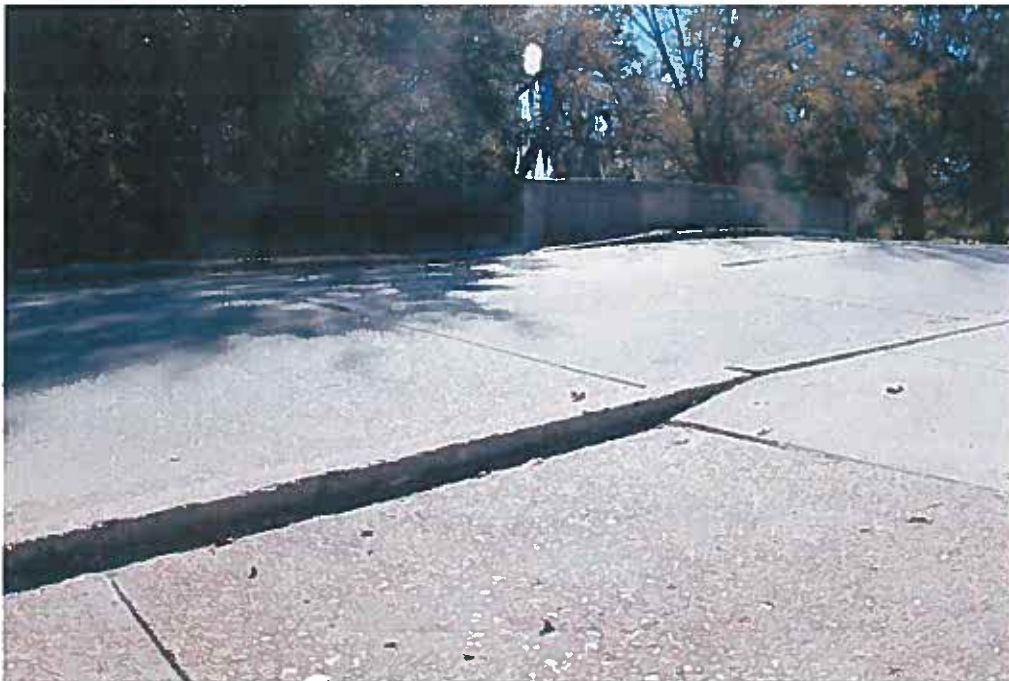
Condition Photo 19: Unsealed joints and settlement of roadway slabs at ends of Recall No. 102235, typical each end.
