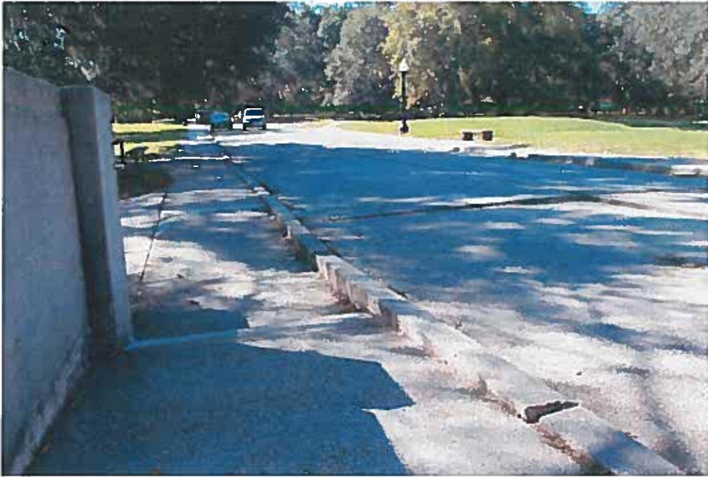
Condition Photo 18: Unsealed joints and settlement of sidewalks at curb line of Recall No. 102235, typical each side of the bridge.
