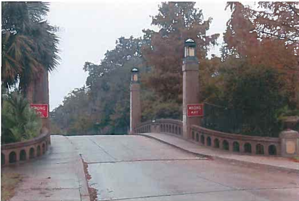
Condition Photo 11: Broken glass in northwest lamp post lantern on Recall No. 102227; condition of lights in four corners of the bridge is unknown.
