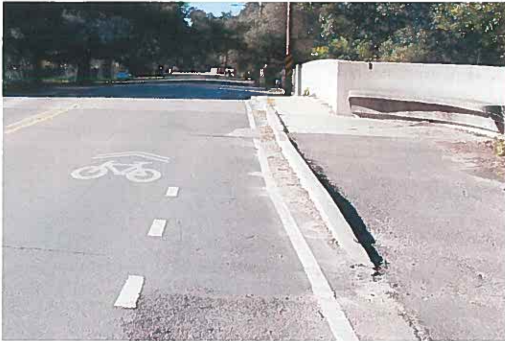
Condition Photo 8: Sidewalk settlement at curb line of Recall No. 102114, and asphalt sidewalk approach settled at curb line resulting in uneven joints.
