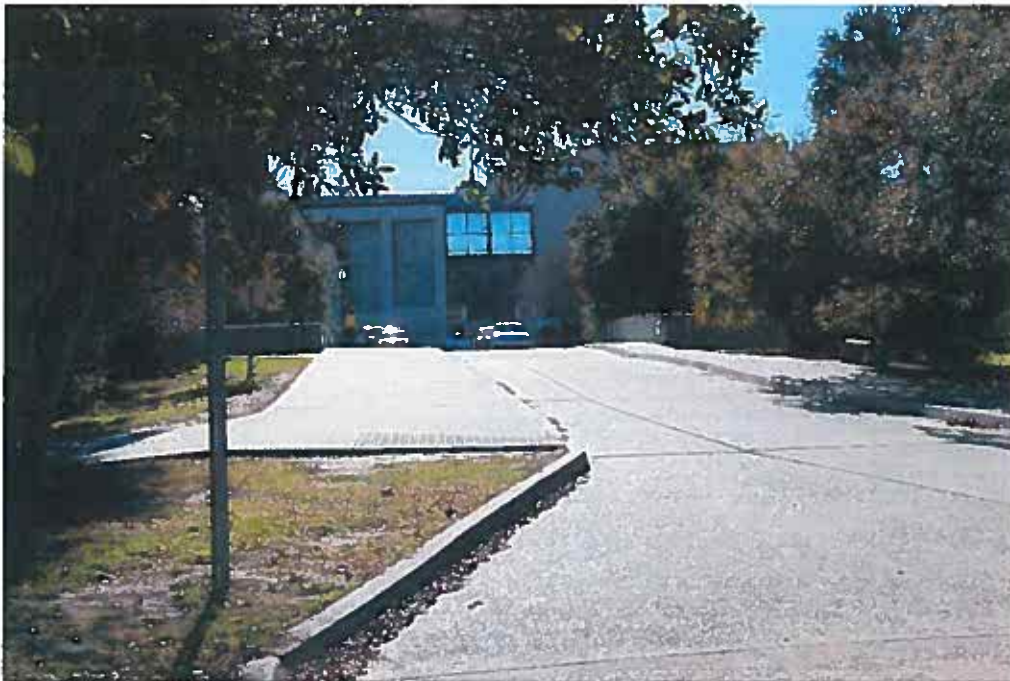
Condition Photo 15: North approach roadway of Recall No. 102233 with unsealed jointed pavement.
