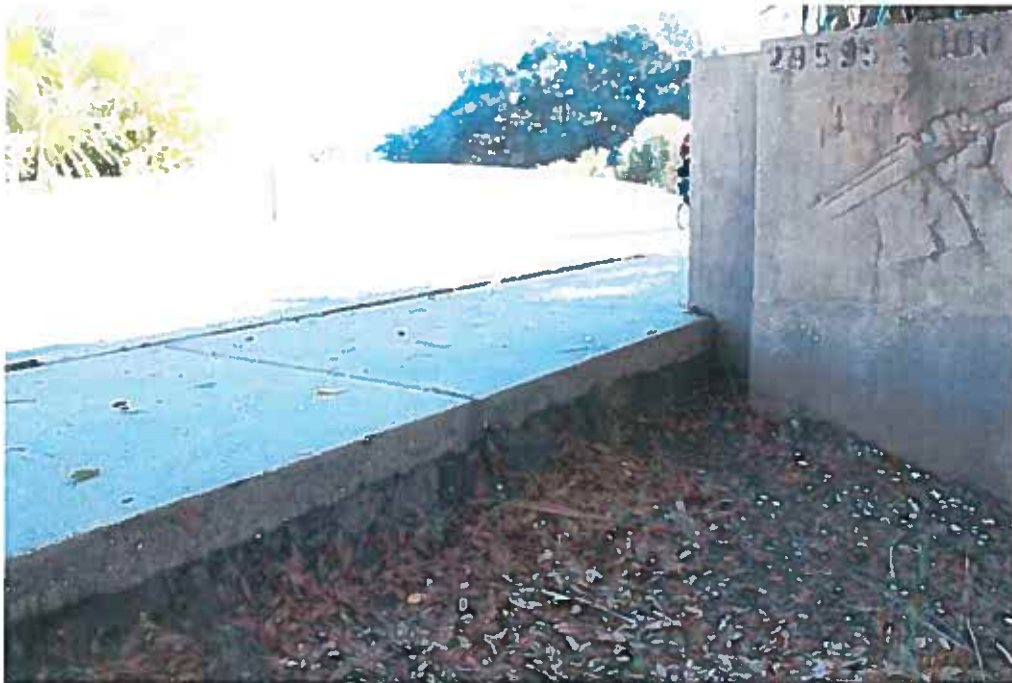
Condition Photo 21: Erosion in southwest corner of Recall No. 102236 at sidewalk, typical on all four corners of bridge.
