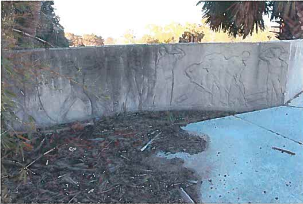
Condition Photo 2: Debris and vegetation accumulation and mold/mildew on concrete surface of bas-relief sculpture (southwest corner of Recall No. 102237 shown).
