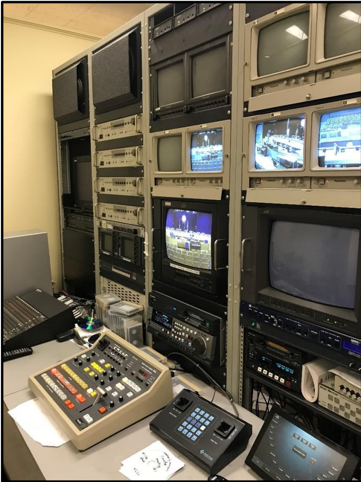
Figure 3: Existing Video Equipment and Controls
