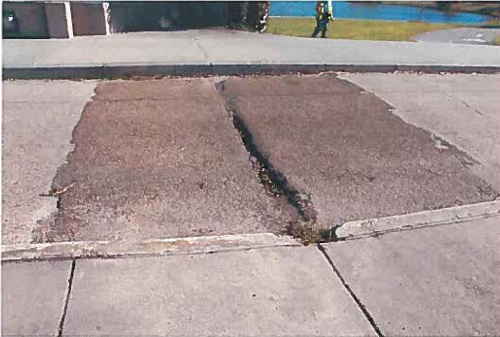
Condition Photo 14: Deteriorated and failed roadway pavement at south approach to Recall No. 102233.
