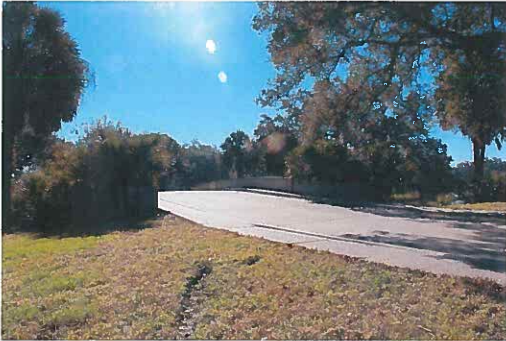
Condition Photo 20: Unsealed joints in concrete sidewalk on Recall No. 102236; settlement at curb line.
