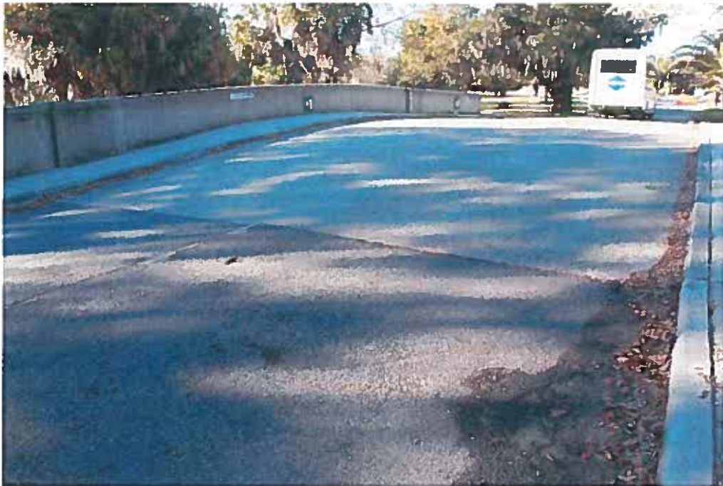
Condition Photo 10: Unsealed joints and cracks in concrete pavement over Recall No. 102226; deteriorated asphalt pavement on easterly approach roadway.
