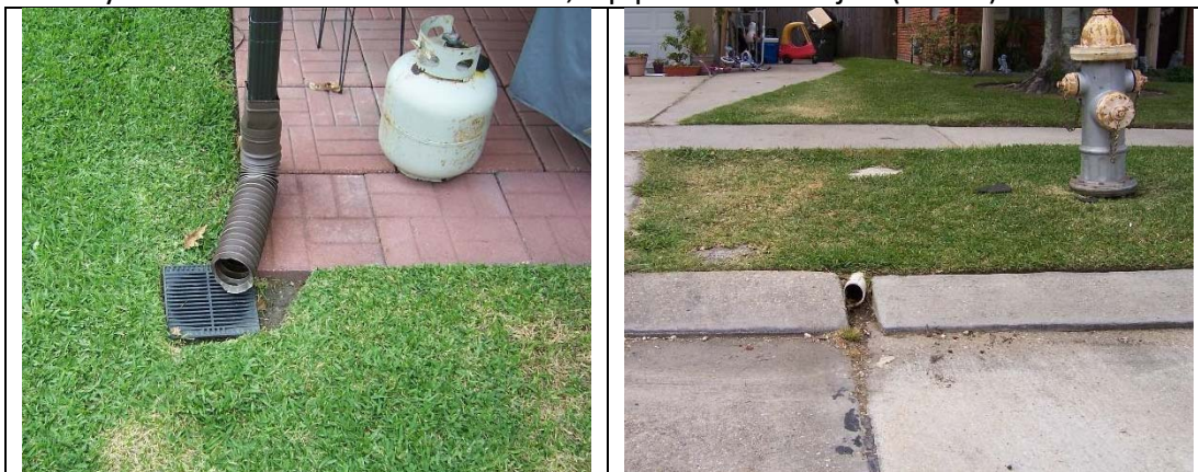
The owner of this house in Jefferson Parish improved the yard drainage by routing roof runoff and standing water to a pipe that runs straight to the street.
