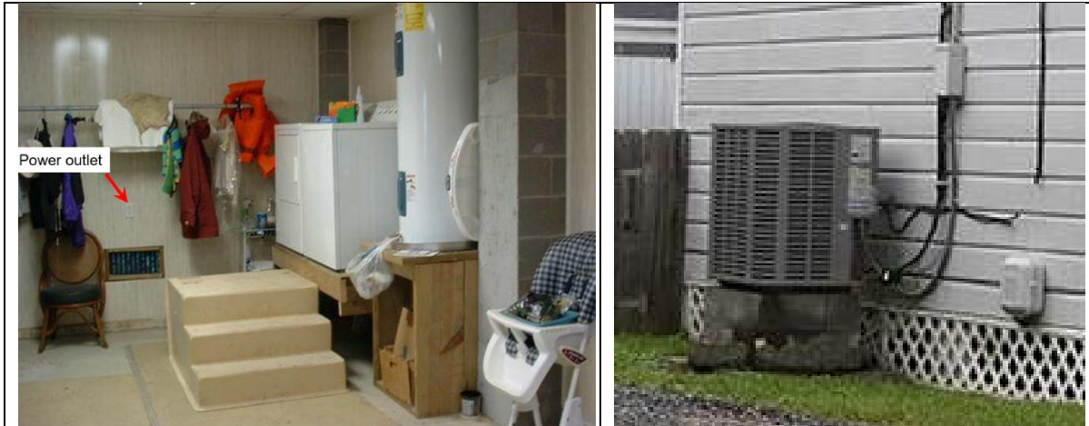
Thousands of dollars in damage can be prevented by simply elevating appliances in a garage or raising an air conditioning unit on blocks, above the flood level.
