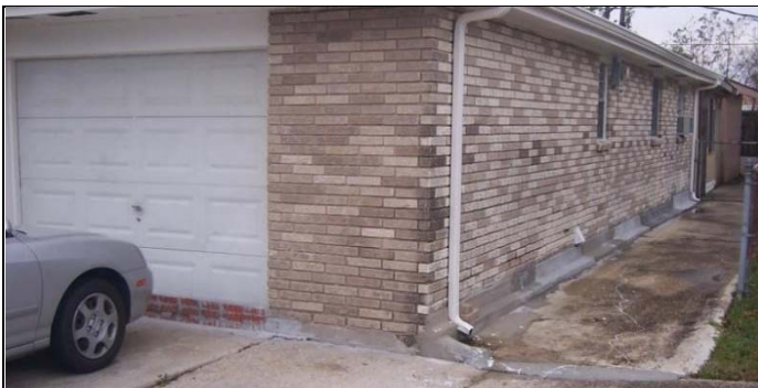
The owner of this house sealed the walls with concrete and built a short, sealed brick wall to keep water out of the garage.
