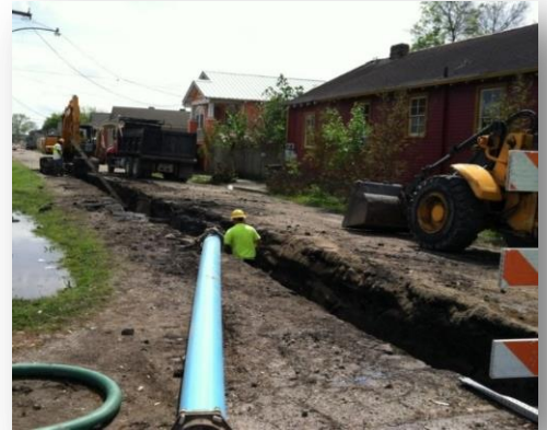
As part of a full depth reconstruction project, contractors will dig a trench similar to the one pictured above in order to replace underground utilities.
