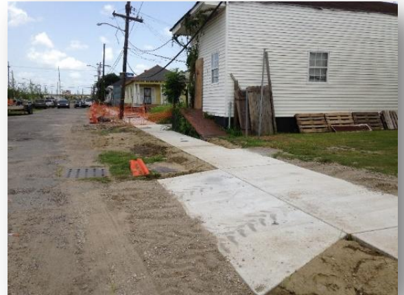
Non-Paving Incidental work is designed to repair damaged sidewalks, driveway aprons and curbs within the public right of way.
