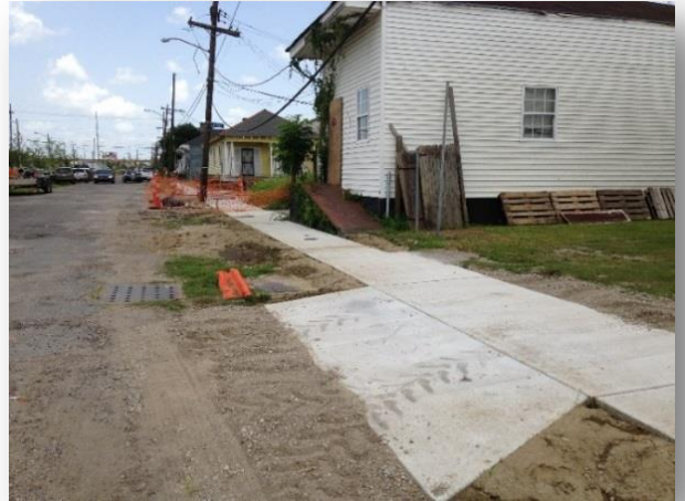
Damaged sidewalks and driveway aprons may be repaired as part of a Patch, Mill and Overlay project.
