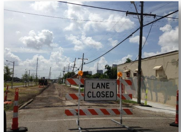
Patch, Mill and Overlay projects are designed to remove damaged portions of the roadway and replace it with smooth new pavement.
