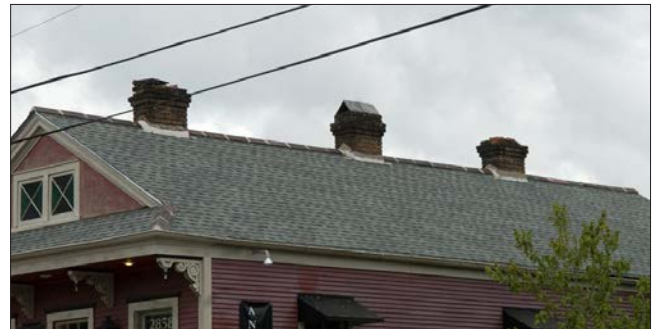
This row of three chimneys suggests the division of rooms on the interior of the building. The central chimney includes an inverted "V" cap and English V ridge tiles with mortared joints marking the top of the roof.
