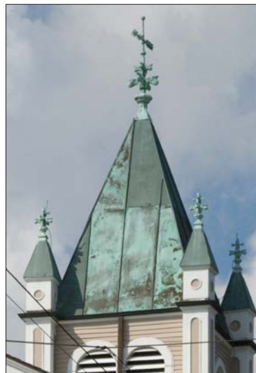
The top of this church tower includes a standing seam copper roof, copper finials and a weathervane. Copper roofing is known for its longevity with relatively little required maintenance.
