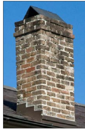
An inverted "V" cap is at the top of the chimney and flashing at its base.
