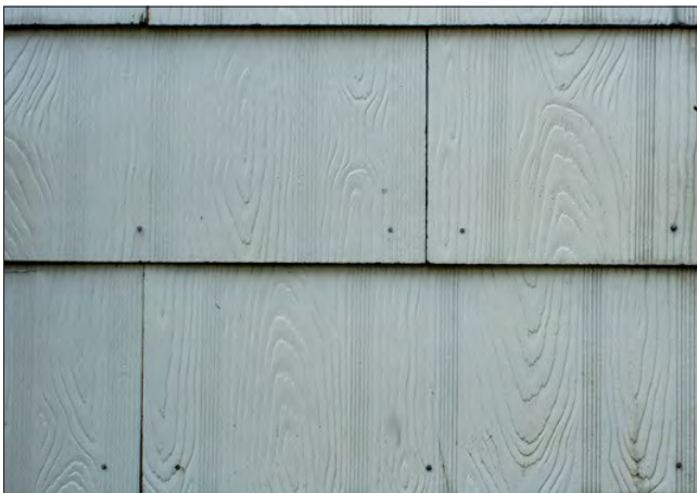
Asbestos siding is often embossed with a wood grain pattern. The removal of asbestos siding can be hazardous and should be undertaken by trained professionals.
