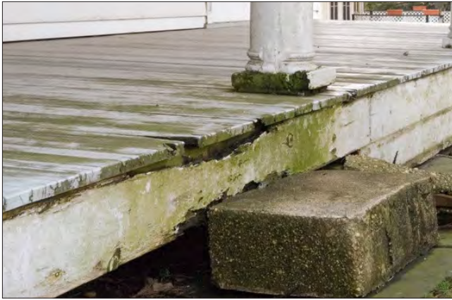
Porches, galleries and other areas where the woodwork is laid horizontally or located close to the ground are often first to deteriorate. Ongoing exposure to moisture can lead to rot of the column bases, porch deck and apron.
