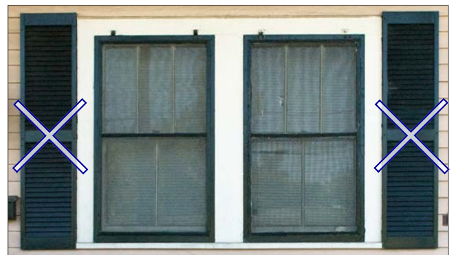
Paired windows rarely have shutters. These shutters are screwed into the wall and would not fit over the window if closed and are obviously fake.
