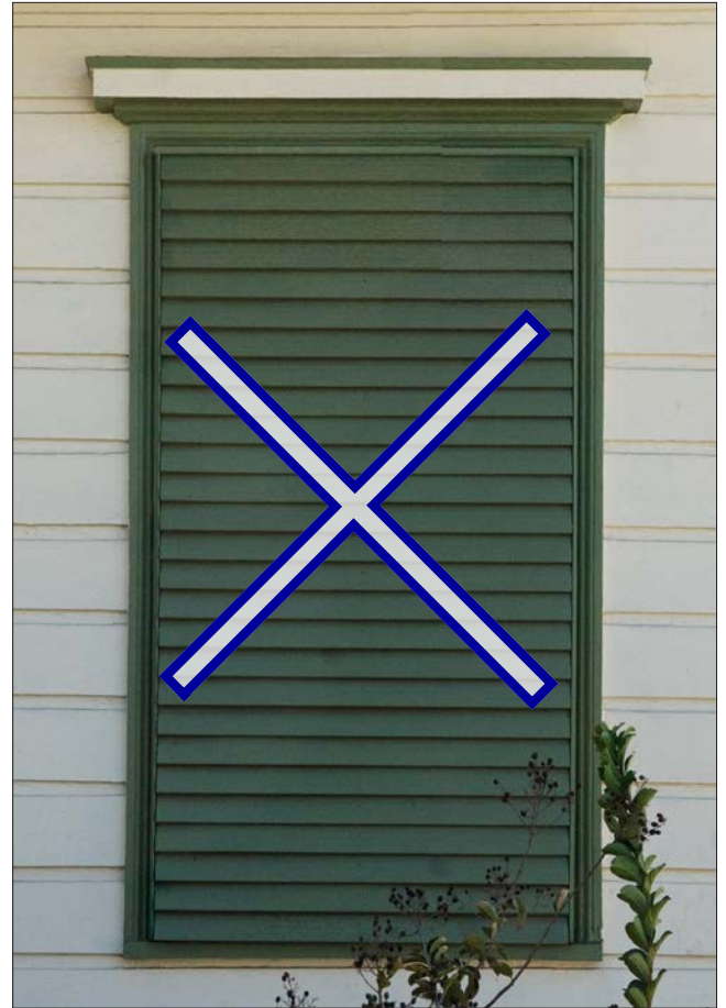
Hurricane shutters should not be permanently installed on windows. They should be stored and installed when needed for storms.
