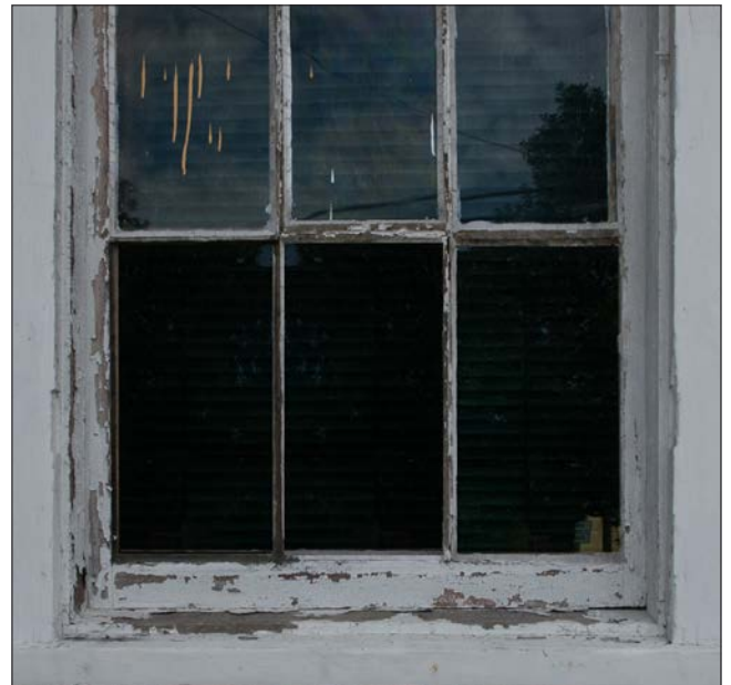
Typically, window deterioration first occurs at the sill. Peeling paint can allow moisture to enter wood and cause rot.
