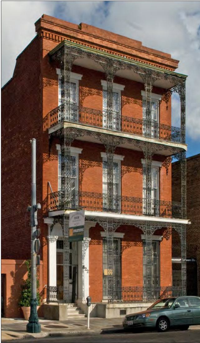
This triple gallery has delicate and ornate cast iron railings, posts and lintels. Note the vent opening at the chain wall.
