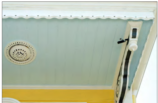
Security cameras, fans and lights should not obscure or be mounted to decorative elements such as brackets and soffits.
