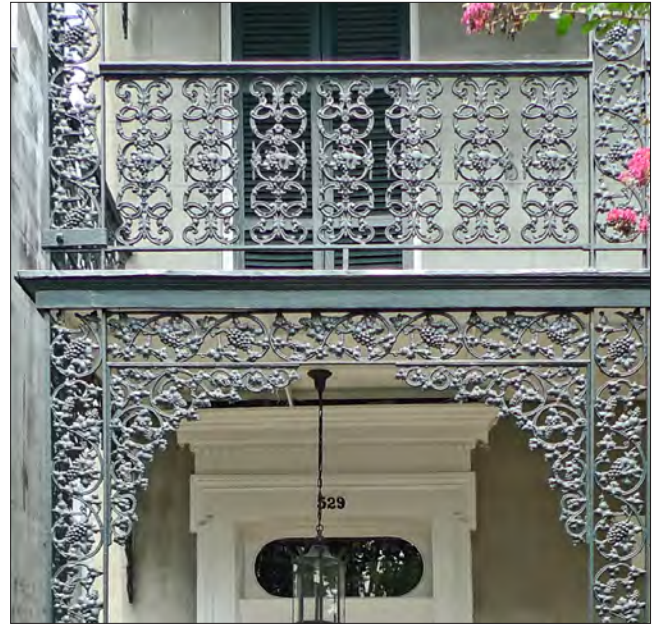
The ornamental metals at this gallery have a motif of grapes and vines. They can be found in the vertical and horizontal supports, brackets and railings.
