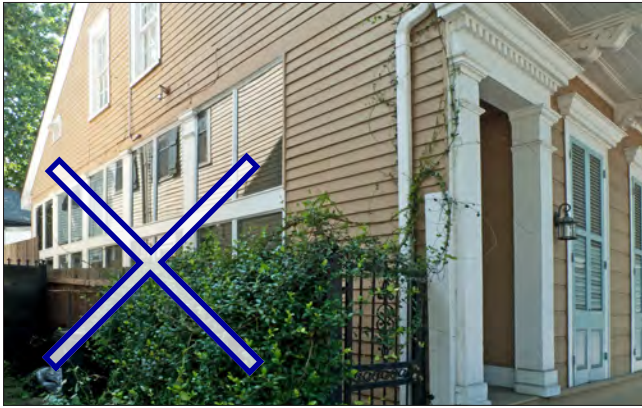
This side gallery has been enclosed with a glazed wall. The HDLC prohibits the enclosure of galleries and porches.
