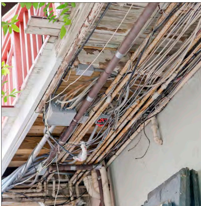
The addition of more conduit, wiring and piping is both unsightly and a potentially hazardous. The visibility of exposed building infrastructure should be minimized and abandoned equipment removed.
