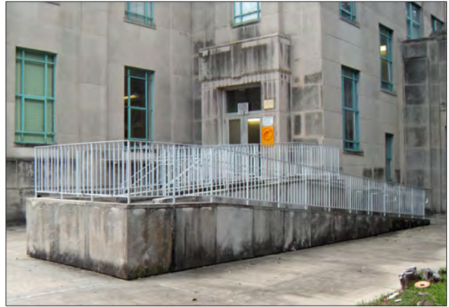
Schools and other institutional buildings will often include ramps for accessibility. The limestone base matches the building and the railings are simple.
