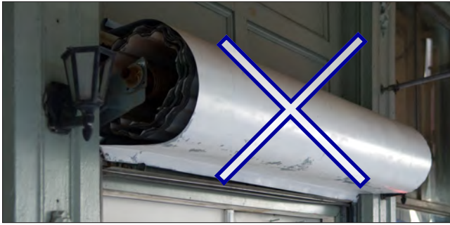
Exterior security grille housings are not permitted.
