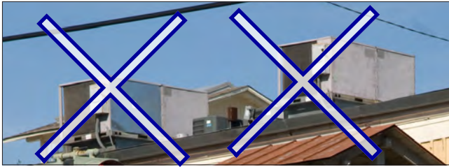
Rooftop mechanical equipment should not be installed in a visually intrusive manner.
