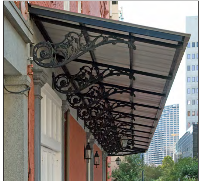
Decorative cast iron brackets and a frame support tongue and groove decking with standing seam roofing above.
