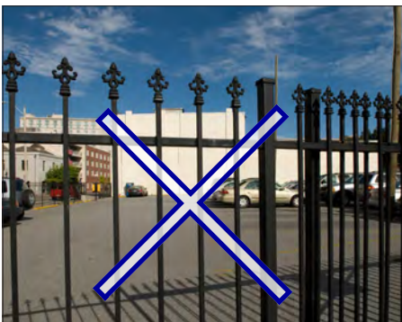
The fence around this parking lot has hollow metal pickets mounted to the outside face of the horizontal rails. Vertical pickets should be solid and pass through rails.
