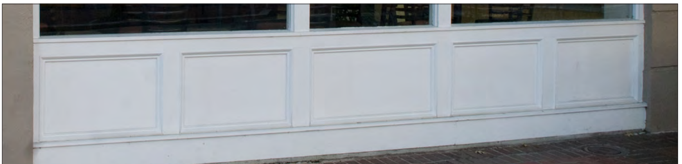
The vertical mullion divisions in the window above correspond to the wood panel divisions at the bulkhead below.
