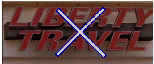
Exposed raceways for channel letter signage are not permitted.
