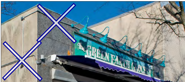
Conduit should be concealed and not mounted to the face of the building. The number of lamps should be reduced to provide enough light for the signs to be read.
