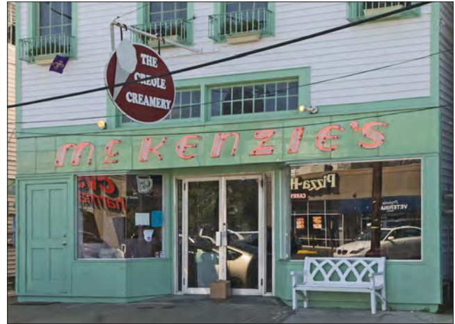
Although not stylistically compatible to the wood framed building, this Vitrolite glass storefront has gained historic significance in its own right and should be retained. Vitrolite is no longer manufactured and there are few remaining examples in New Orleans. The new store owners have retained the historic signage and added a new projecting sign.
