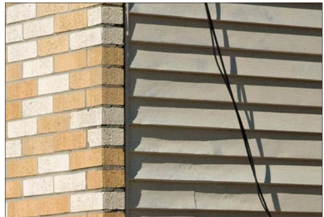
The left wall of this wood framed house has been covered with brick veneer. The addition to the right has been covered with vinyl siding. Both are inappropriate materials and should not be utilized in historic buildings.
