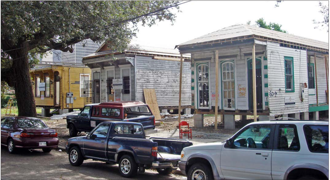
These Side Gallery Shotgun residences have been saved from demolition and moved to a new location. The entrance porches and roofs will be restored to prepare the homes for new families.
