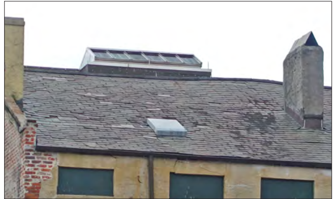
Deteriorated roof conditions ay dramatically increase the vulnerability to storm damage of a building.
