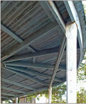
The framing and tongue and groove boards are clearly visible at the underside of this canopy that is supported by chamfered wood posts. Note that the locations of the posts align with the corner of the masonry building.
