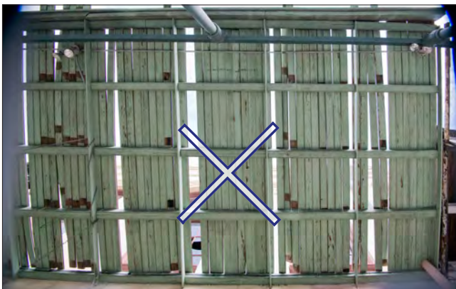
Several floor boards from this gallery are missing and loose. The remaining boards may fall onto pedestrians or become airborne in a high wind. Immediate repair is recommended.
