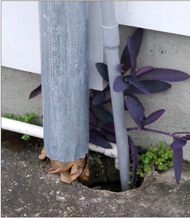
The downspout is clearly clogged with leaves and is discharging onto the sidewalk instead of into the drain. It is likely that the clogged downspout will overflow onto the building walls.
