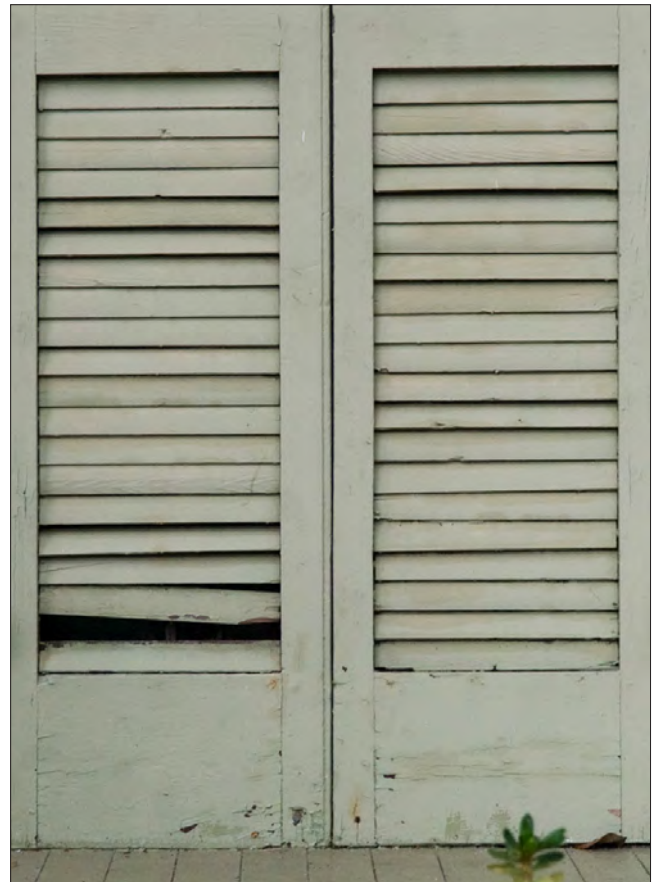
The broken and missing louvers on this door shutter can be repaired and/or replaced in-kind, allowing it to remain on the building and continue to function. Regular repainting will minimize the potential for rot.
