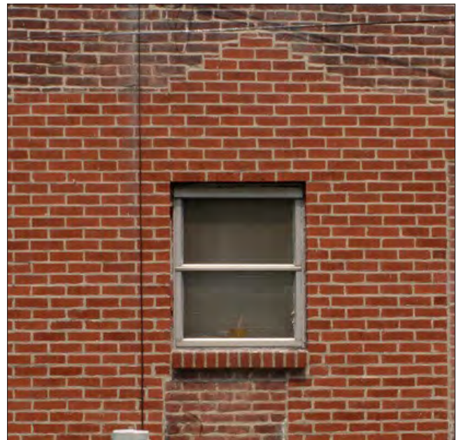
Masonry infill areas – The brick infill area is clearly visible. The infill area uses bricks of a different size and color than the historic bricks and is outlined by a thicker mortar joint rather than being “keyed” into the adjacent brickwork.
