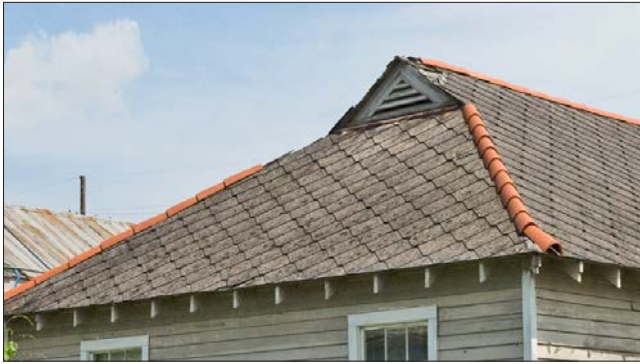
The asbestos shingle roof has terra cotta caps on the ridge and hips and a triangular louvered vent at the front gable. The ridge caps and louvered vents should be retained. Gutter installation is recommended.
