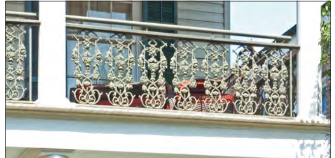
A higher secondary safety rail has been installed behind the cast iron balustrade to meet code requirements.
