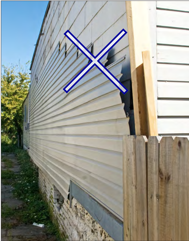
The vinyl siding has been partially removed. If not repaired, the remainder of the vinyl is likely to be pulled off in hurricane strength winds. Asbestos shingles are visible under the vinyl, which are likely covering wood siding. Complete removal of vinyl and asbestos siding, and restoration of wood siding is recommended.
