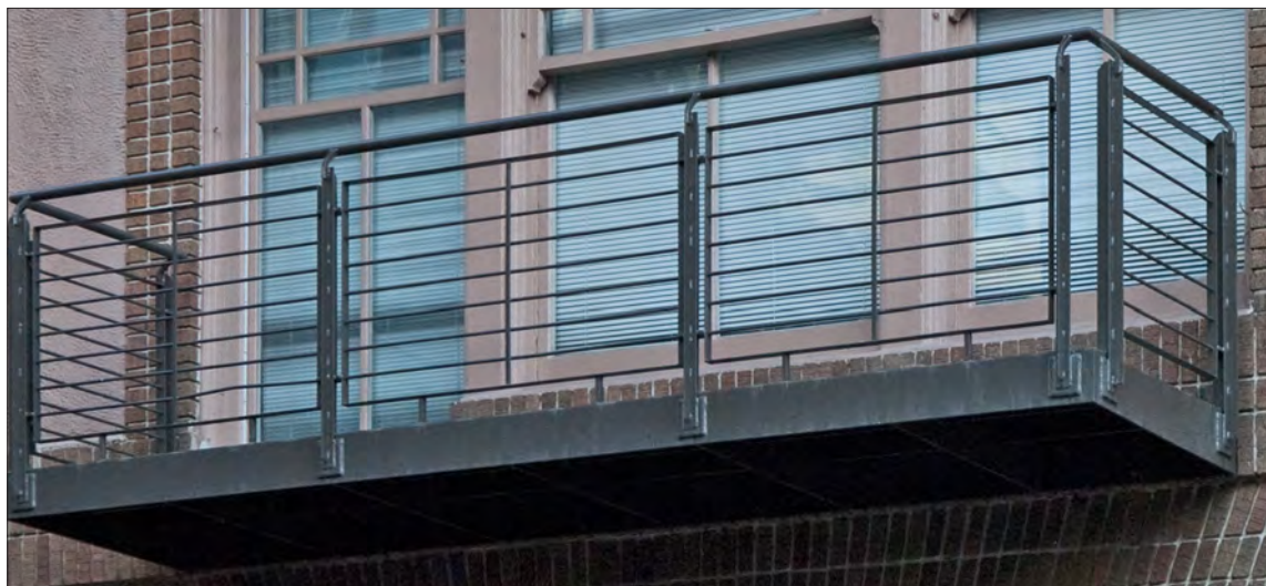
This balcony appears to “float” in front of the window and is fastened to the wall at the platform level.
