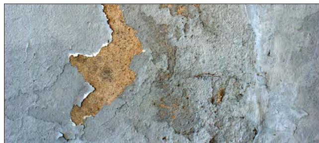
The peeling paint is likely incompatible with the stucco or caused by moisture. Loose and flaking paint should be removed and the cause for failure addressed before repainting.
