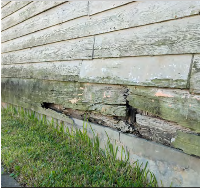
Wood located on or next to a brick or a concrete foundation or pier is more likely to absorb moisture and rot as well as attract termites.
