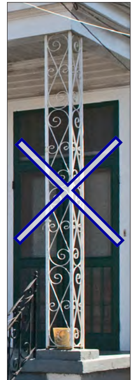
Modern Metal Post Not Permitted
