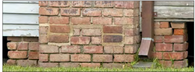
Regular review of piers can alert property owners to when joint repointing or repair is needed.
