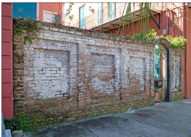
This brick wall has a decorative pattern that suggests panels and piers. The rear yard gate is located within the arched opening.
