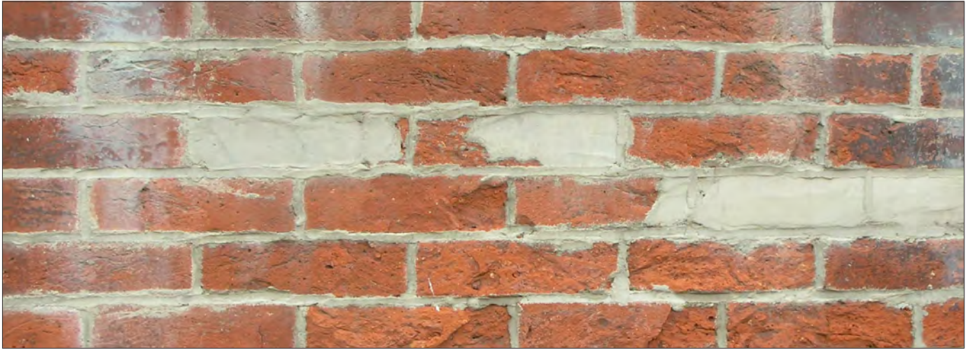
The rough texture and uneven surface suggest that an aggressive cleaning method was used. Stucco patches replace bricks and efflorescence, a white powdery substance, can be seen on the surface.
