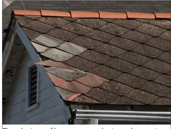
The asbestos roof has some non-asbestos replacement shingles of a similar size and shape as the existing roofing.
