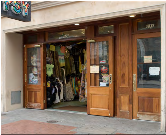
A new wood storefront was installed that includes transom windows, sidelights, glazed paired entry doors and a secondary door to access upper building levels.
