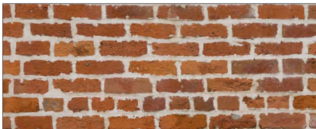
Widened and extended joints – A power tool was used to cut-out the joints during repointing, extending vertical joints. The joints have also been widened and are too large.
