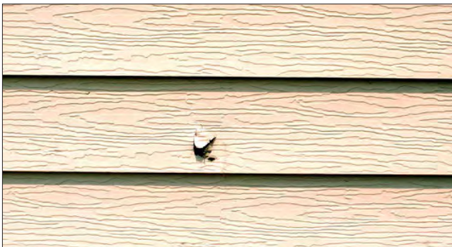
Replacement of this aluminum siding section would be the best way to repair the puncture. Since siding colors tend to fade from sunlight, the replacement siding probably would not match the existing adjacent siding.
