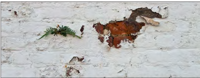
The peeling paint is likely incompatible with the brick or may be caused by moisture. The plant growth indicates moisture trapped in the wall. The paint should be removed.
