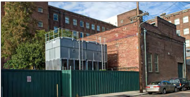
This HVAC equipment is located within this building's courtyard, partially concealed by a fence at a secondary street elevation. It would be preferable if the height of the equipment was lowered to the fence height to minimize visibility.
