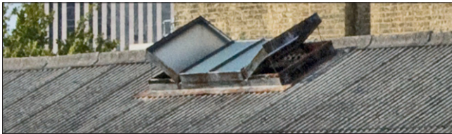
Some skylights were historically located in warehouse and commercial buildings, providing natural interior light and ventilation. The visibility of new skylights should be minimized.
