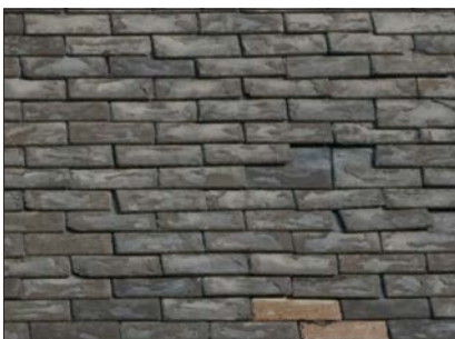
Individual missing or damaged slates can often be replaced, extending the serviceable life of the roof and postponing costly replacement.
