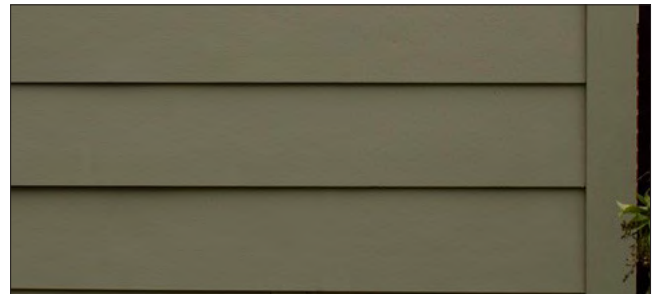
Fiber-cement siding material is a good economical alternative for new construction or an addition to a historic building. It can be painted to match the existing paint scheme.
