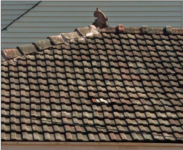
This concrete tile roof includes a finial and terra cotta ridge caps at the top of the main roof and along the roof hip.
