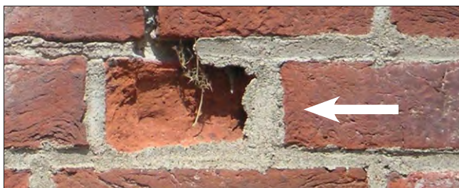
Spalling of the masonry surface – The center brick surface has spalled. The repointing mortar likely includes too much Portland cement and is harder than the bricks. The mortar should be removed and replaced with soft mortar.
