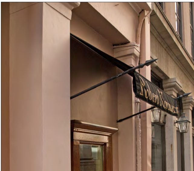
The awning is mounted between the granite piers. The poles are fastened to the stucco surface rather than the masonry, facilitating future repair if removed.
