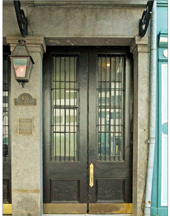
The granite lintel is structural, spanning between the flanking Greek Revival pilasters.
